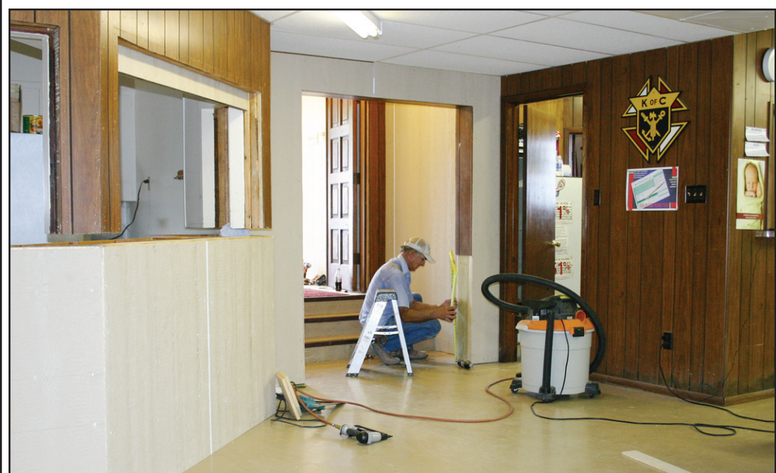
A work in progress, as repairs and upgrades, inside and out, at the Muenster Knights of Columbus Hall continue. Pictured is Bill Bayer working on the downstairs entry. The Muenster Knights will be celebrating the 75th "birthday" of the KC Hall this Saturday, hosting a party for everyone to attend. Janie Hartman photo
