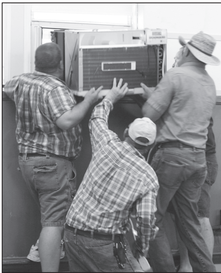
A crew of Ernie Martin, Paul Fleitman, Bob Knauf, and Karl Koesler places a new air conditioner in the fourth grade classroom at Sacred Heart in preparation of the first day of school next week.
