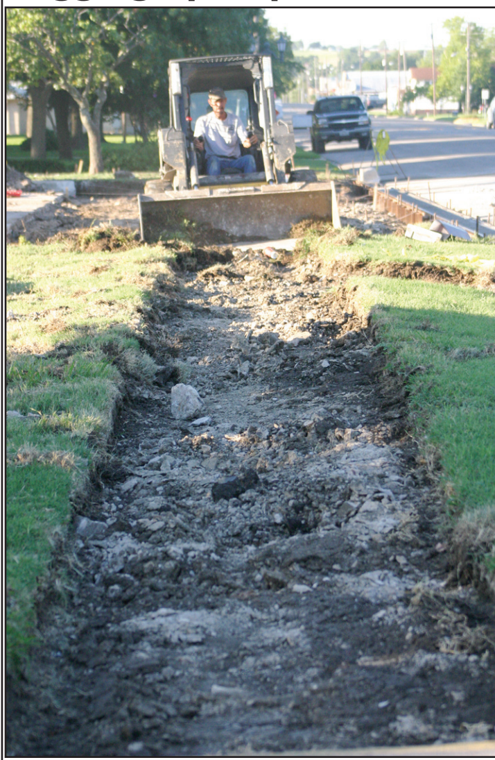
The Dangelmayr Construction crew took out the sidewalk along Main Street in front of the Sacred Heart Community Center. A new sidewalk will be constructed along with an enlarged entry into the parking lot. Janie Hartman photo
