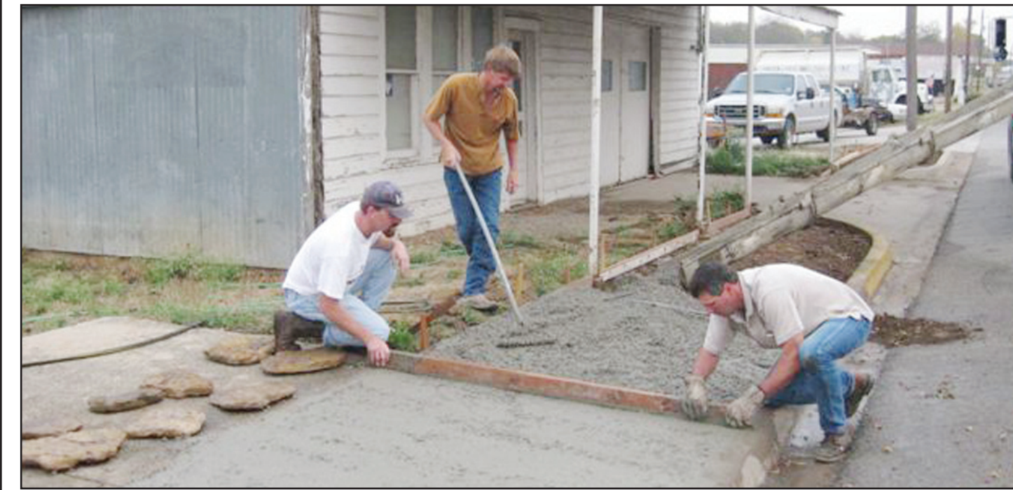
This is the work which is being done by Fischer's Meat Market as part of the KMB project "To the Curb and Beyond." Cement was poured and rocks donated by Johnny Rohmer were placed into the cement. Doug Fleitman also donated some rocks and spent time with a helper troweling the cement. Pictured are, from left, Kelly Bob Bayer, Doug Fleitman, and Steven Fisher. The parkway is on Third Street in front of a lot and building which was often overgrown and violated City ordinance because it is considered no-mans-land and not kept by anyone. Steven Fisher took it upon himself to remove the parkway, and cement and rock it at his own expense. KMB photo
