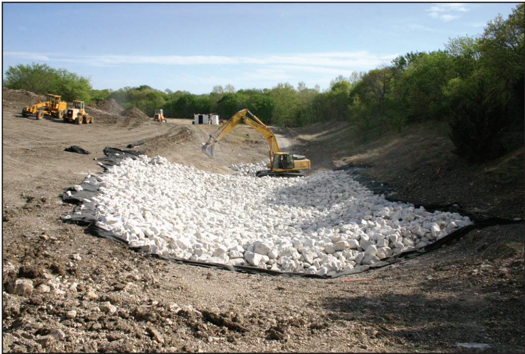
Heavy rains in 2009 caused considerable damage to Johnson Lake's spillway. It is a flood control lake and dam located northeast of Muenster. In a cost share program between Cooke County Precinct #4 and the U.S. government, major repairs are being done to the auxiliary spillway. More than 100 trailer truckloads of large rock were hauled in and placed to prevent future erosion and damage to the auxiliary spillway. Janie Hartman photo
