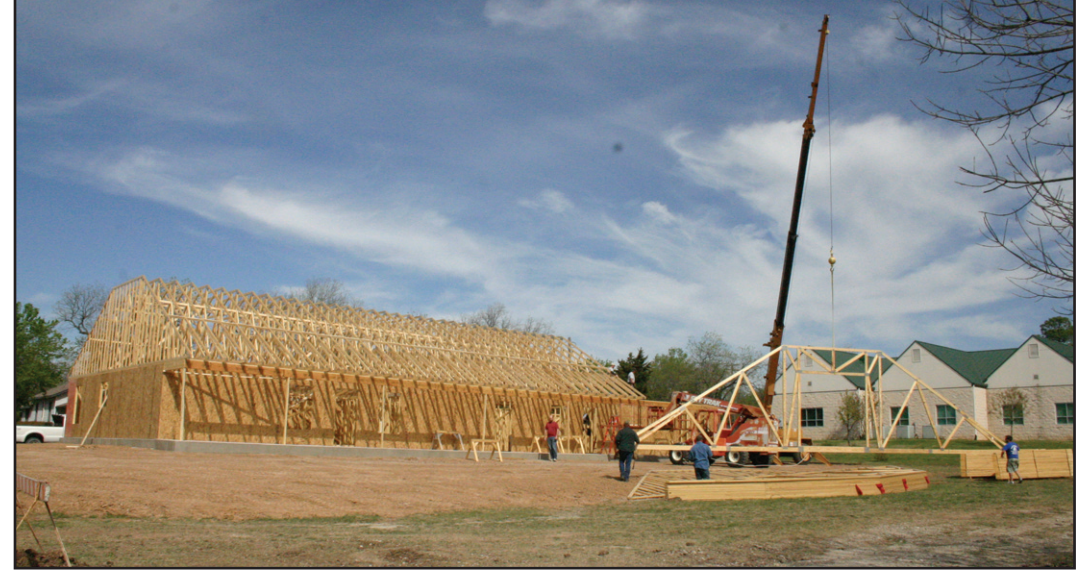
Framework progresses quickly for a daycare center on North Elm Street, one of the new businesses being built in Muenster. Janie Hartman photo
