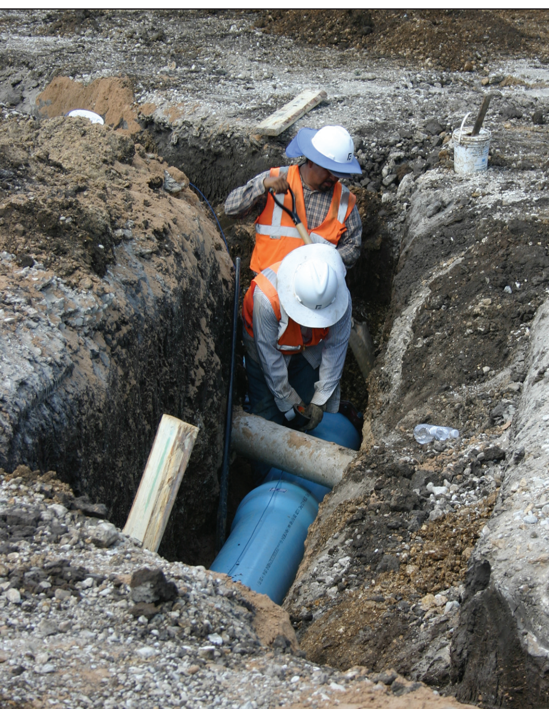
Work continues on Muenster's new waterline coming from the new 200,000 gallon storage tank. The new (blue) 12 inch line crosses under the old 6 inch line in the 200 block of South Main Street. The City is laying 8,700 feet of new pipe, connecting this line to the 12 inch line at Hwy. 82. Janie Hartman photo
