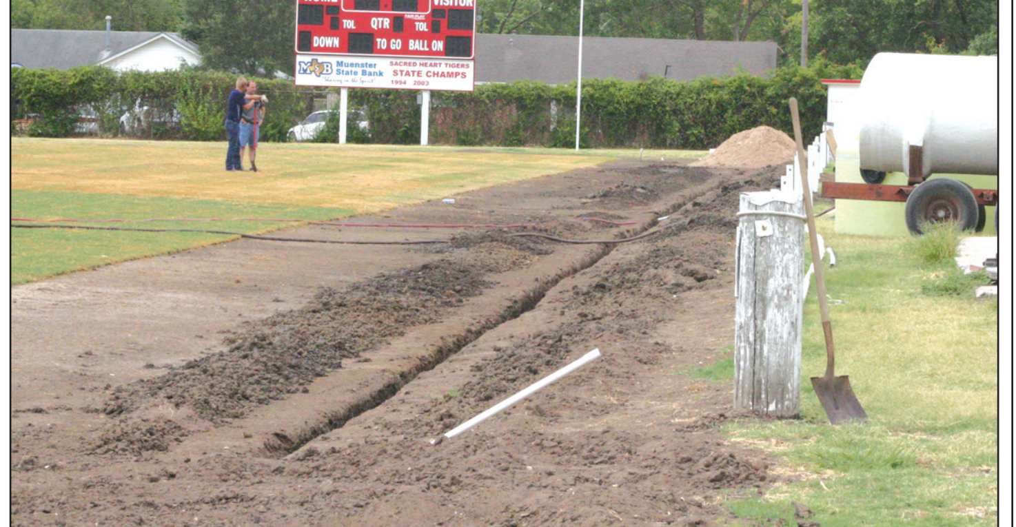
Improvements to the Sacred Heart Tiger football field continue in preparation for the upcoming season. With the extreme heat and hard rationing, tanks of water are kept on site to allow sufficient watering of the newly installed grass. A hardy grass called Celebration was planted and, according to school officials, should be ready for the upcoming football season. Janie Hartman photo
