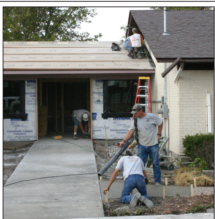
Dangelmayr Construction, D & B Construction, and others continue work on the expansion of the Sacred Heart Montessori building this week. The project will not be complete for opening day.
