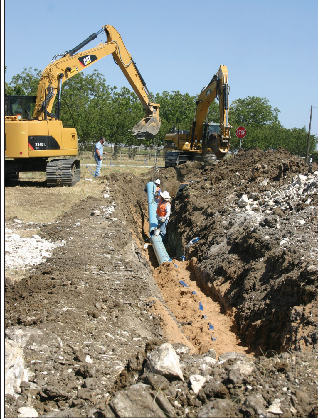
Muenster's water improvement project is in its final stages. A 12-inch water line is being laid along FM 373 north of town that will connect with the six-inch line that now serves the Sicking subdivision. There have been problems with water pressure in that area and it is hoped that this new line will improve both the pressure and volume of the water. Work on the water line is being done by Fain Group of Fort Worth.
