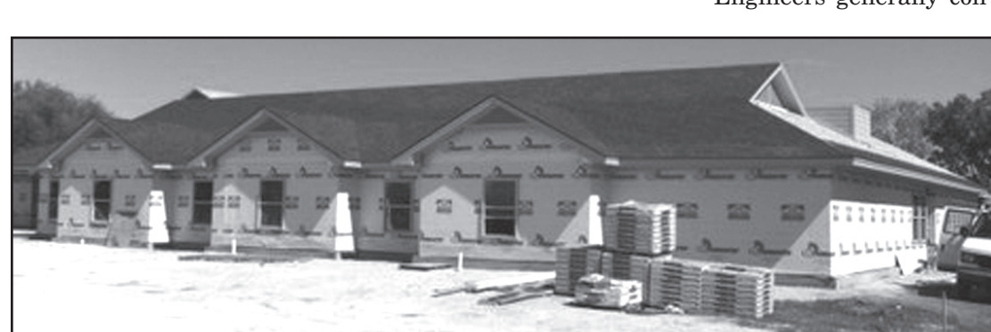
Abigail's Arms shelter, pictured at left, continues to take shape in the form of brick and mortar, shingles, windows, and doors, and will stand as a fortress to help protect victims of domestic violence. While the structure is vitally important - what will take place inside is crucial. With caring volunteers and staff, the shelter will be able to provide a refuge for their clients as they move on to self-sufficiency and a life free from abuse. Visit www.abigailshelters.org to make a donation. Courtesy photo
