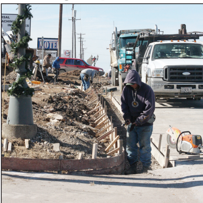
The crew from Huchton Construction put in curbing along Highway 82 in front of Universal Machining last week, an improvement towards the beautification of Muenster.
