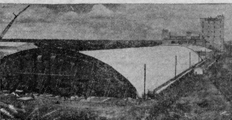
WORLD'S LARGEST AIR SUPPORTED BUILDING erected this week in Fort Worth by a grain handling firm, as it appeared before and after four giant fans lifted the 2.3 acre 50 ton steel roof 38 feet from ground level. The job was completed in 10 hours. More than 1,800,000 bushels of grain will be stored in the air-tight, cement-floored building.
