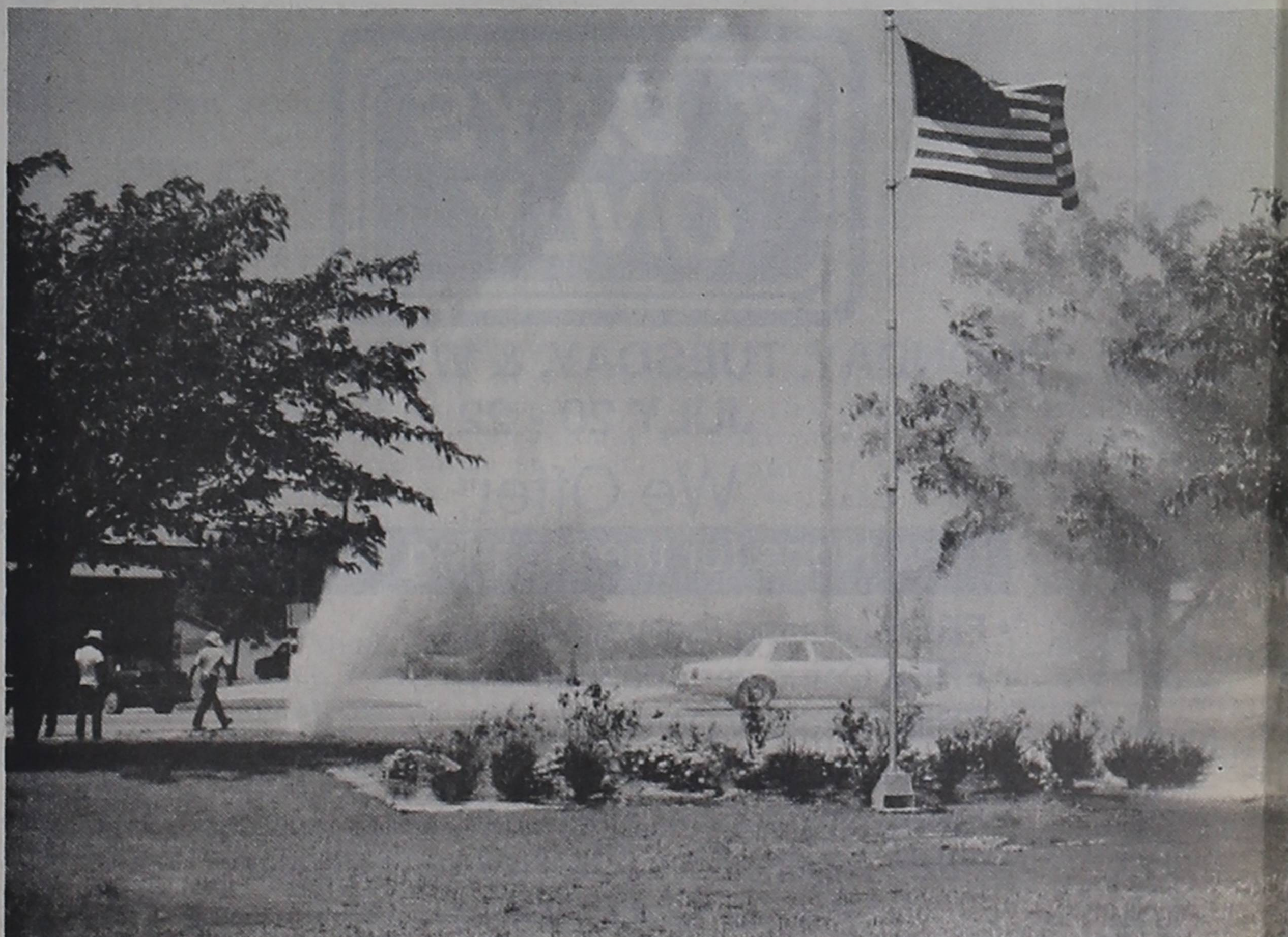
MUENSTER had its own geyser for a short time last Thursday. The impressive sight was created when a break in a water line on Main Street near Mid-Park ripped a hole in the pavement and drenched the area with water. The break occurred while city employees were working on faulty water lines near City Hall. Janet Felderhoff Photo
