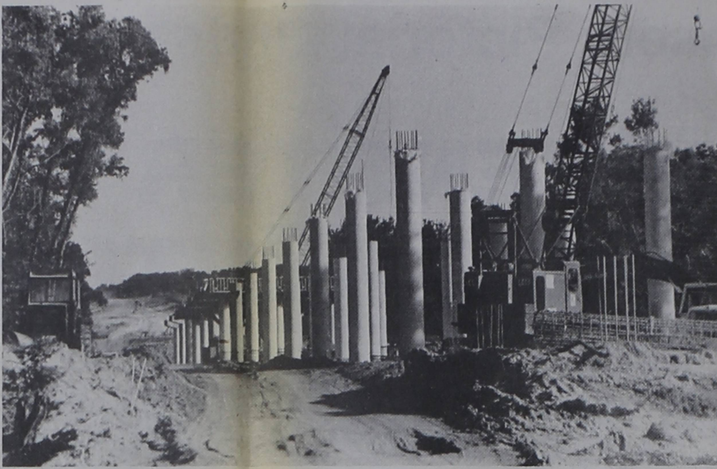
CONCRETE COLUMNS stand in pairs awaiting completion of a new bridge that will connect Texas and Oklahoma near the towns of Courtney, Oklahoma and Illinois Bend. Virgil Hess, Precinct 4 commissioner, has county workers constructing fences along roadways in the county that will eventually provide access to the new bridge. Janie Hartman Photos
