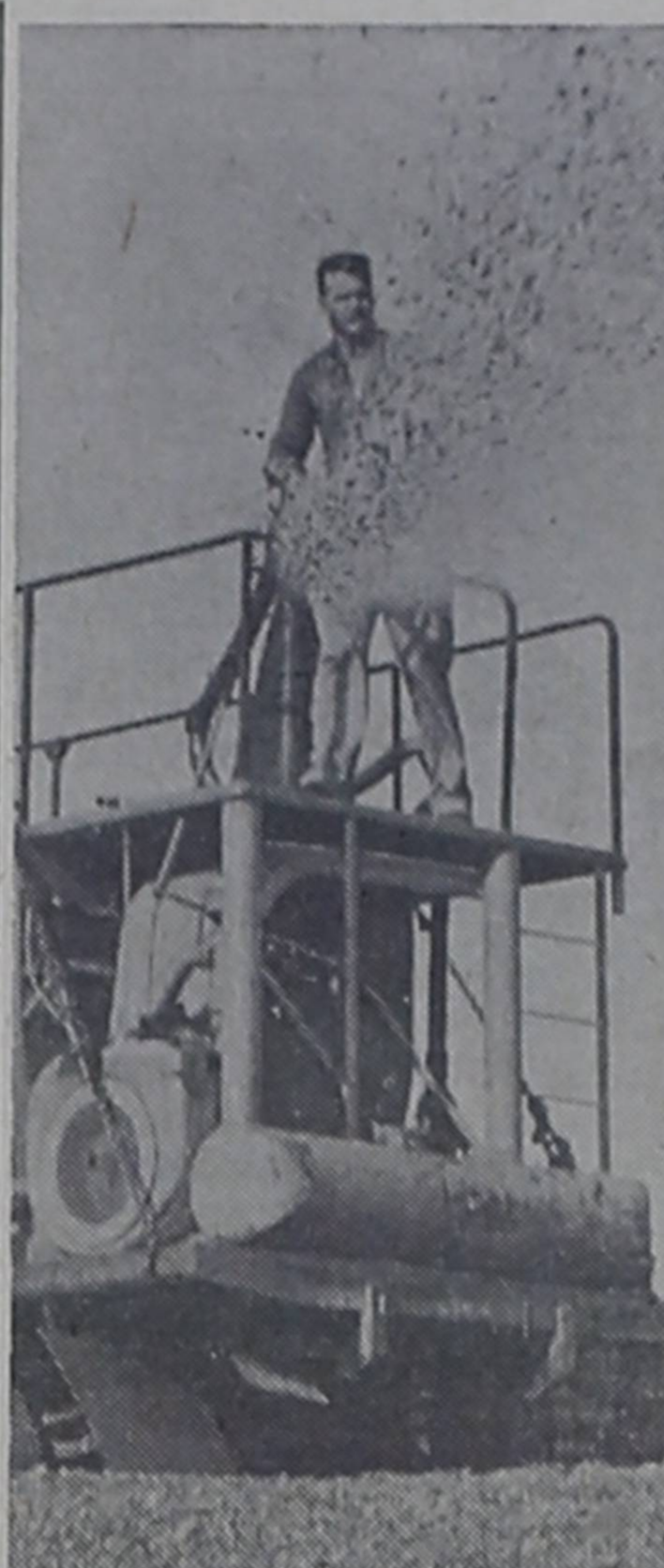
SEED SPRAY —Large turret gun mounted on truck shoots out a seed mixture in a new method used to plant grass near San Antonio, Tex. Spray mixture contains special wood cellulose fiber mulch to hold the grass seed in place.
