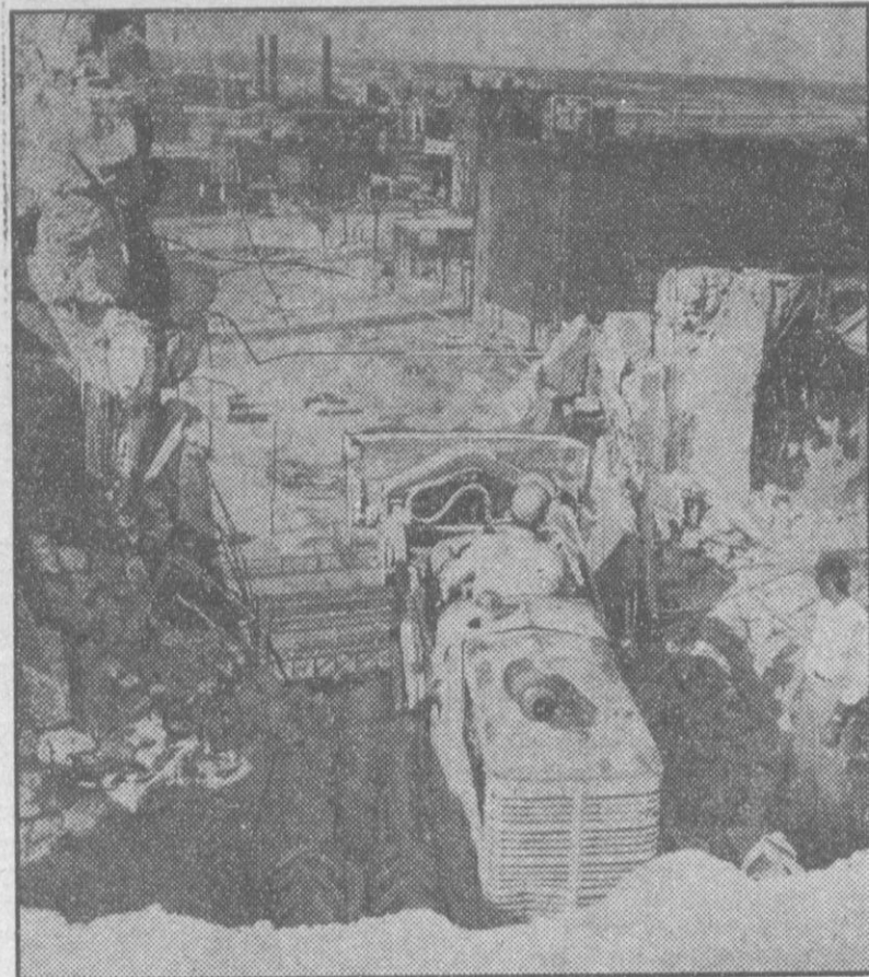
NO DOZING ON THIS JOB —It takes a wide-awake operator to "dig" a bulldozer through an 11-story building from the roof to the basement. The 19,000-pound machine was assembled atop a building being wrecked in Kansas City, Mo., and used to push debris over the side of the structure as it was demolished, floor by floor.
