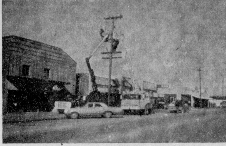
Electric service lines in Muenster are being modernized by the TP&L maintenance crew.
