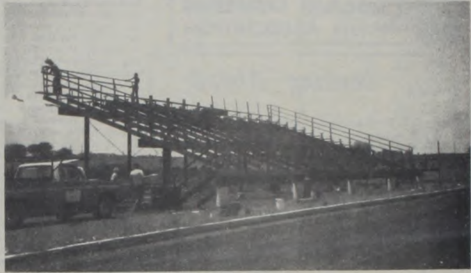
Construction of the home side grandstand at the new Hornet football field and track got under way last week after months of delay by wet weather. The steel structure with aluminum seats and stairs will seat 750 persons.
