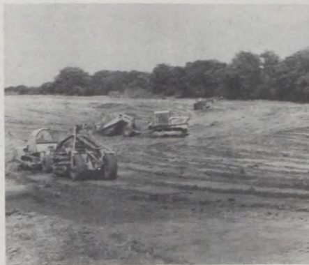
Construction of grade stabilization structure on Norris Dill farm. It took about 15,000 cubic yards of earthfill because the gully was so large.
