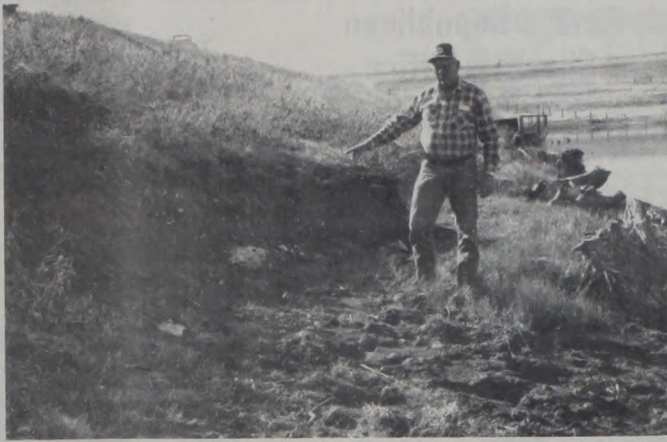
Picture 1 J.H. Bayer points out erosion damage to front slope of flood control dam caused by wave action.
