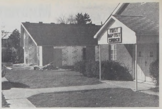
The new First Baptist Church is being constructed along side the old building which will be renovated into a fellowship hall. Staff Photo
