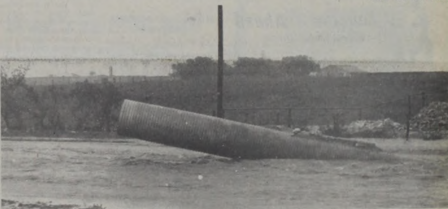
Swirling floodwater dislodged this culvert on Mesquite Street during Tuesday's flood. Janie Hartman Photo
