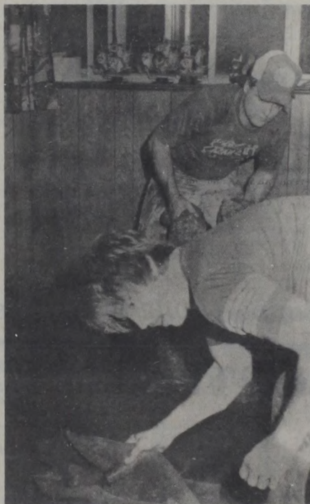
Chris Sicking and Mark Lippe work at the messy job of removing flood soaked carpet and padding from Dan Luke's home Wednesday evening. Staff Photo
