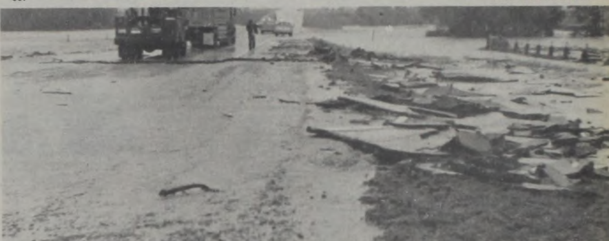
The ravages of Tuesday's flood caused this pavement damage on Highway 82 between Myra and Lindsay. Janie Hartman Photo
