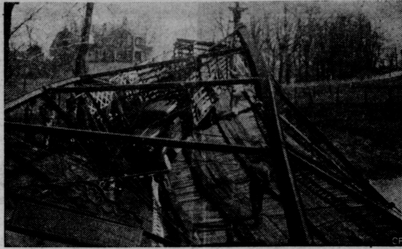
THORNTOWN, Indiana.—One hundred foot span bridge over historic Sugar Creek on Road 47 at Thorntown crushed and tumbled into the creek last week when large stock truck driven by Jesse Wetherald of Thorntown skidded in rain and crashed into a corner support.
