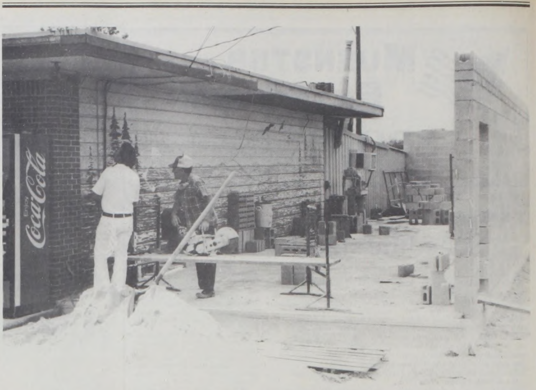
CHAS BAYER and Bobby Lutkenhaus discuss where to make a cut in the west brick wall of Bayer's Kolonialwaren, currently undergoing major construction. While several changes are being made in the interior and exterior of the business, just what the new merchandise will be is a
