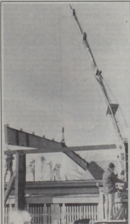
Workmen guide a roof support girder into place at Community Lumber Company, where the local business is remodeling and adding an extension to its main building.
