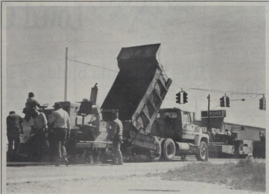
As if cooperating with Germanfest, the Highway Department has finished its repair project on the road into town. Equipment here is applying the last of the surface material.
