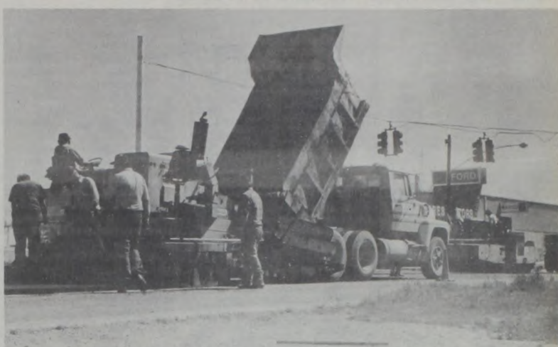
STREET PAVING WAS BIG NEWS through most of 1984 as city and state both got into the act locally.
