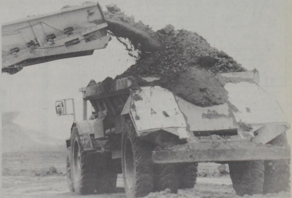
THE BELT LOADER (see front page) fills 45-yard bottom-dump trucks in less than a minute with soil from the lake bottom.
