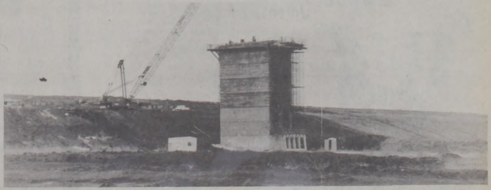
CONSTRUCTION OF THE TOWER dominates the horizon along the three-mile length of the dam, which still has 20 feet to grow.
