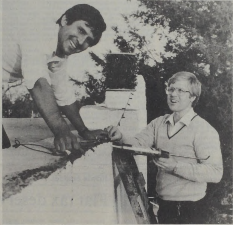
LIGHTING CONTEST CHAIRMAN Gary Fisher, left, helps parade chairman David Fette Tuesday as they test a new technique of anchoring Christmas lights to outline a building. A big effort is set this
