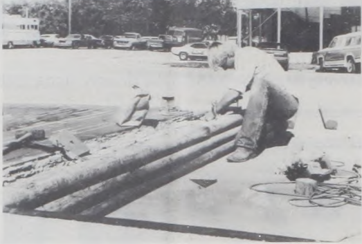
Doug Fleitman works on extensive planter boxes at the vacant AMPI lot. The planters will soon be home for hundreds of flowers in the continuing Muenster beautification and landscaping effort.
