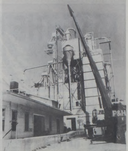
This towering crane has accented the Muenster skyline for the last several days. Muenster Milling Co. is replacing the top of the elevator leg and the turn head which controls the flow of grain to different bins. The old one had been used for 30 years. Janie Hartman photo
