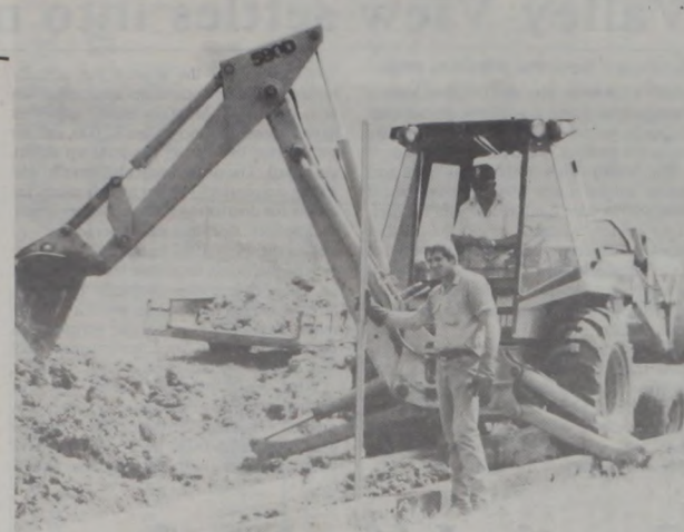
WORKERS CLEAR OUT A DRAINAGE DITCH at the Muenster football field, in preparation for the coming football season which opens in two weeks.
