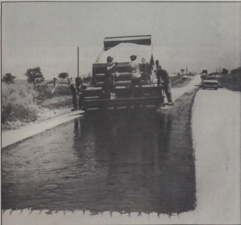
THE DUST PROBLEM is a thing from the past as city and county workers complete the first layer of paving on Ash Street. A second coat will be applied in the near future. Photo by Janie Hartman
