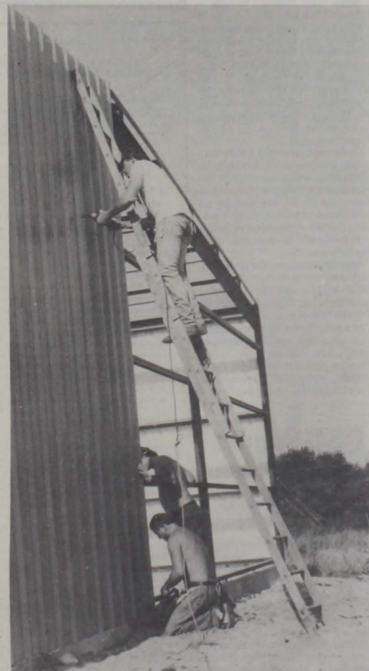
MIKE STURM , co-owner of Muenster Auto Parts, attaches the siding onto the new building going up on West Hwy. 82. Mike and Larry Gobble hope to move Muenster Auto Parts and Muffler Shop into their new location next month. The parts store covers 3,000-square feet with a 2,000-square foot muffler shop in the rear. The new building will allow for a 75 percent larger inventory. Neal Walterscheid and Steve Fette are also pictured working on the new building.
