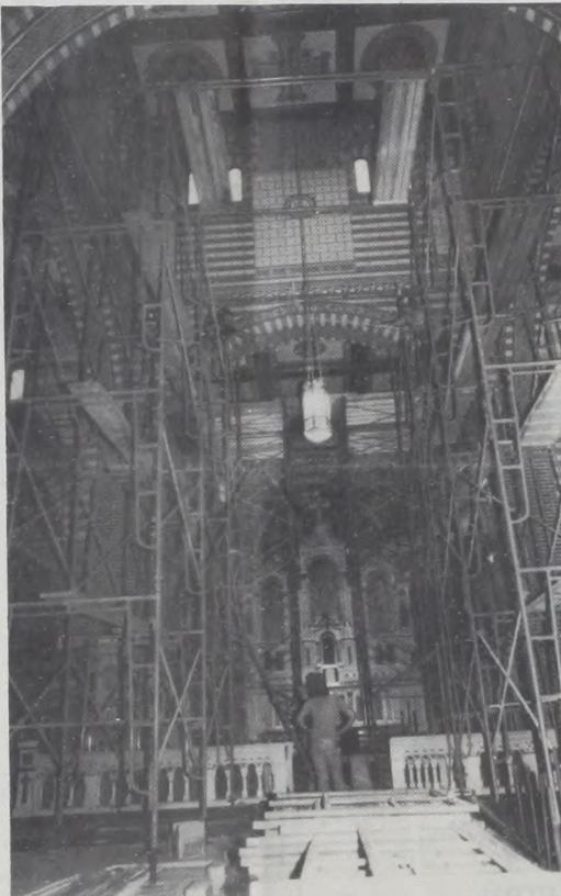
St. Peter's Church in Lindsay started extensive renovation in June. Janie Hartman Photo
