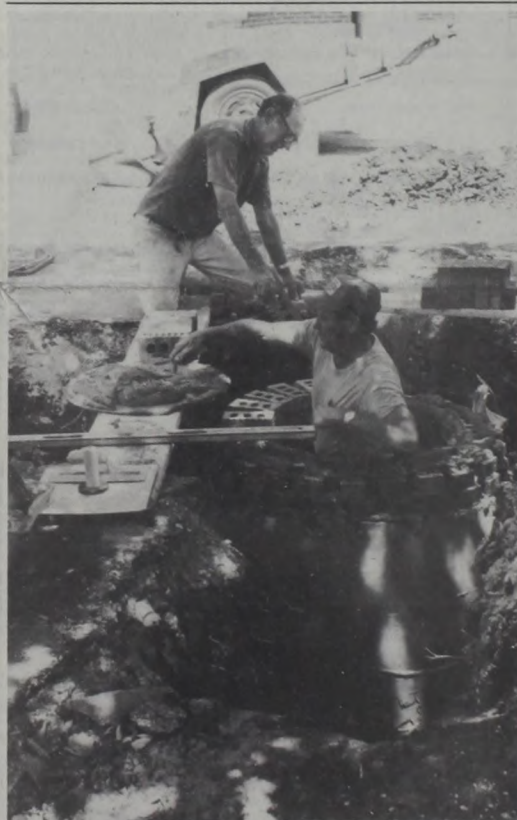
EIGHTY-TWO FEET of drainage pipe was replaced this week on Sacred Heart Parish ground. The old original pipe collapsed behind the church, causing backup in the church basement. Pictured: Bobby Lutkenhaus assists Robert Klement in constructing a manhole in front of the grade school for easy access to the pipes in the future. There was no damage to the church basement or its contents.
