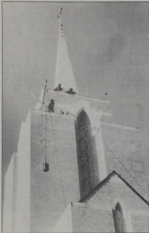
WORKMEN REPAIR the tar and gravel roof walkways on the steeple of Sacred Heart Church last week. All flat surfaces on the church were resurfaced along with the roof of the annex which forms a second story over the garage of the rectory and the gymnasium. Janie Hartman Photo
