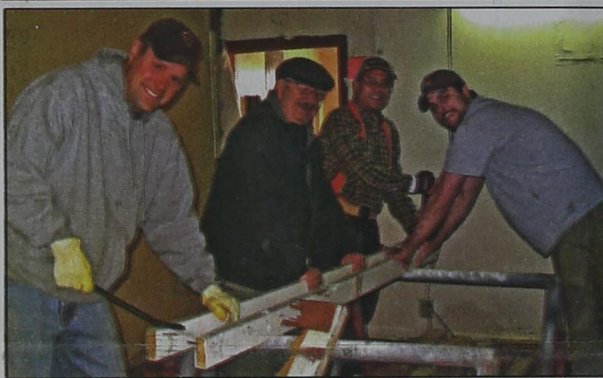
Ryan Davis, Cecil Biggers, Tindle Ramon and Mickey Schoenhals work on building shelves for the new Hansford Food Pantry, located at 210 Main Street in Spearman. Cecil has donated the use of his building for the Food Pantry, and members of Methodist Men scheduled a work day on Saturday, March 27th. Other volunteers helping, but not pictured, were Randall Sauer, Mark Schoenhals, Robert Howell, and Dallasene Reynolds. Another work day will be scheduled in the near future. If you would like to make a donation to the Hansford Food Pantry, or would like more information, please call 806-659-5531.
