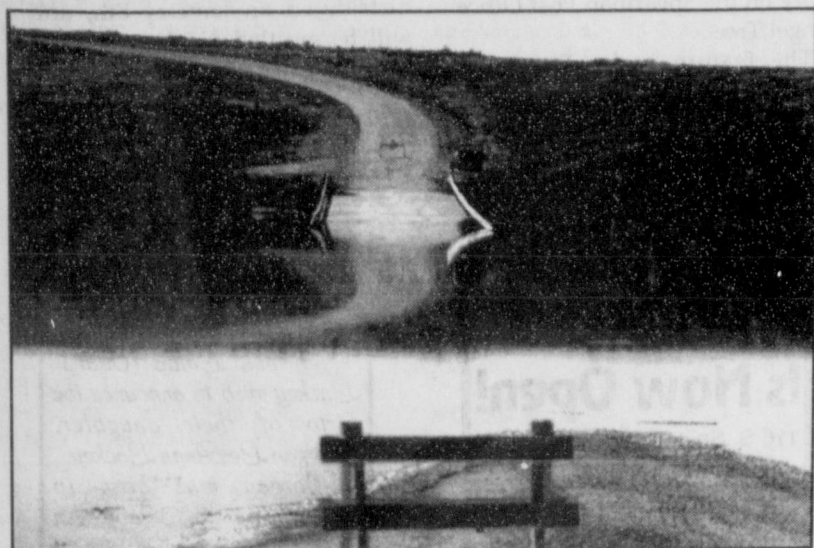
Pictured above is a view of the lake at the Palo Duro Creek Bridge. The water is still 2-2 1/2 feet over the Highway.
