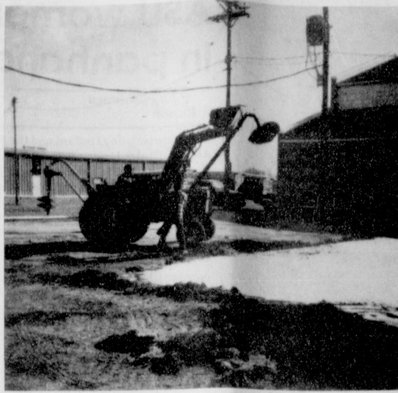
Two men work to complete the cement slab on the Gruver playground project.
