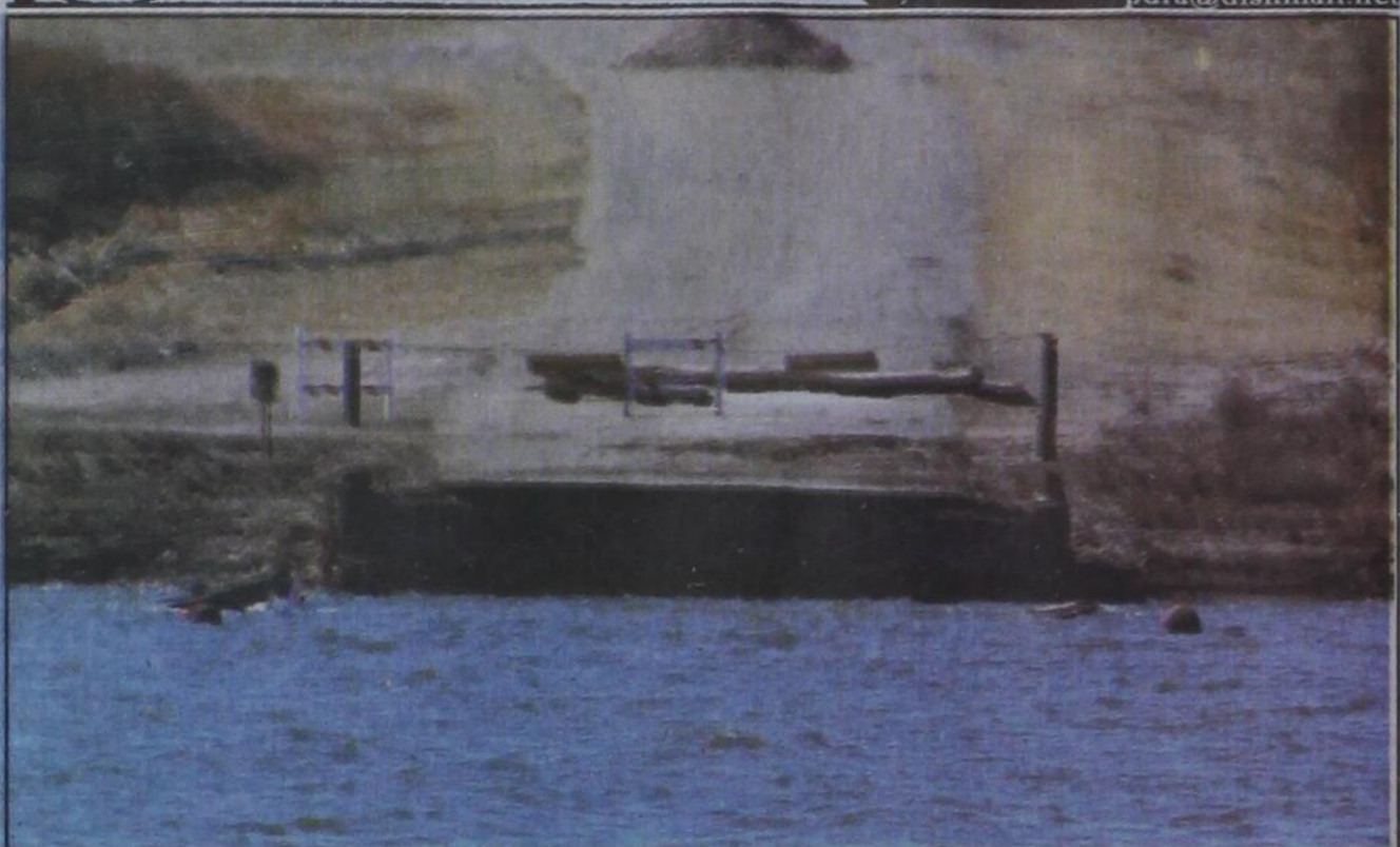
This is a picture of the Palo Duro Creek bridge, at Lake Palo Duro. It washed out in mid June 2010 flood.
