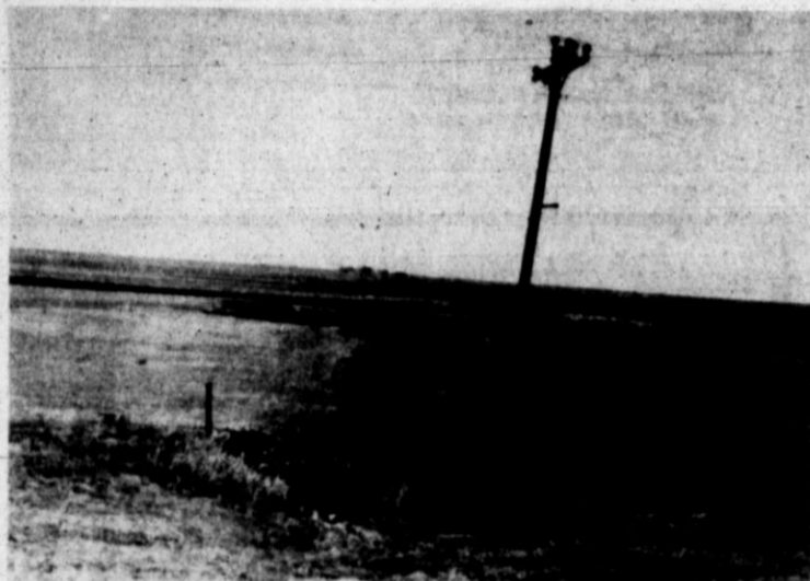
THE BEFORE — Steady run off onto a portion of the A. C. Hays ranch northeast of Hereford created this huge gully big enough to park a school bus in. The run off also was causing erosion of the county road.
