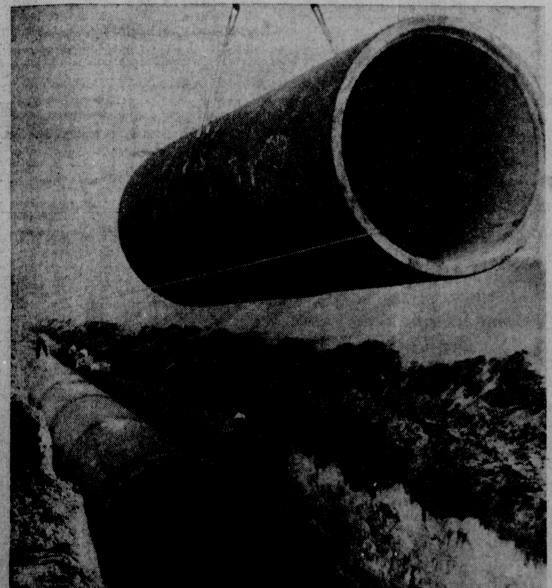
Workmen on the Canadian River Aqueduct southeast of Amarillo prepare to receive another 22-foot joint of the massive pipe and place it in position. This particular
