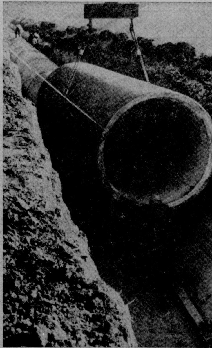
Despite its girth and weight, a joint of the huge pipe is a relatively simple object to handle when swung into place by a crane. One man here guided a joint to its destination in a pre-shaped hole formed by another machine operating some 75 feet on farther down the hole.
