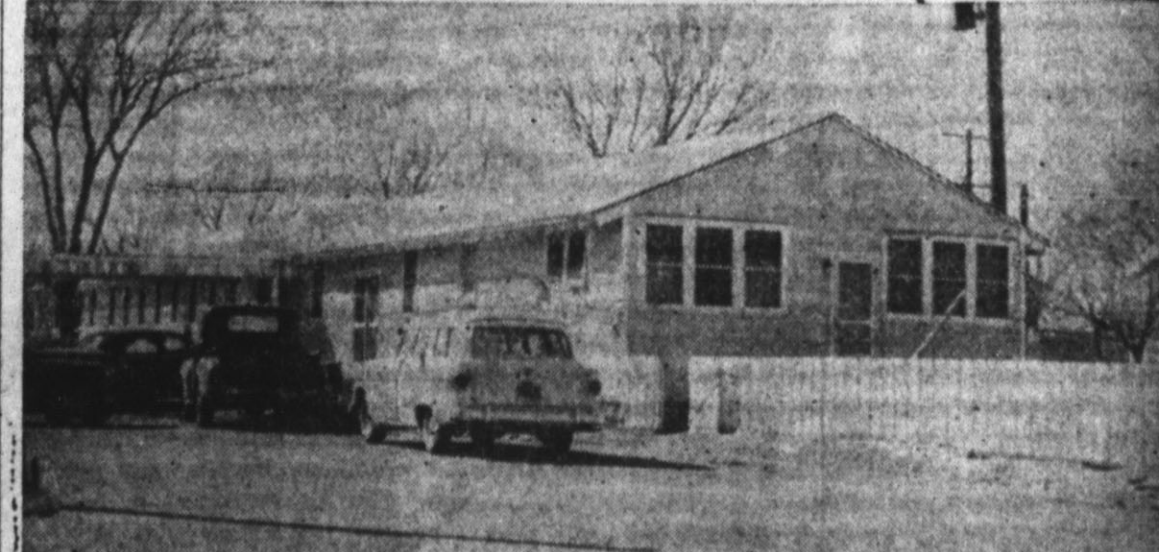
WORK BEGINS —Work got underway last week on the new Deaf Smith County Hospital nurses home. In the picture at top, workmen begin getting the groundwork done. By Saturday concrete forms were going into place. The picture below shows the present barracks being used for a nurses home. (Staff Photos)
