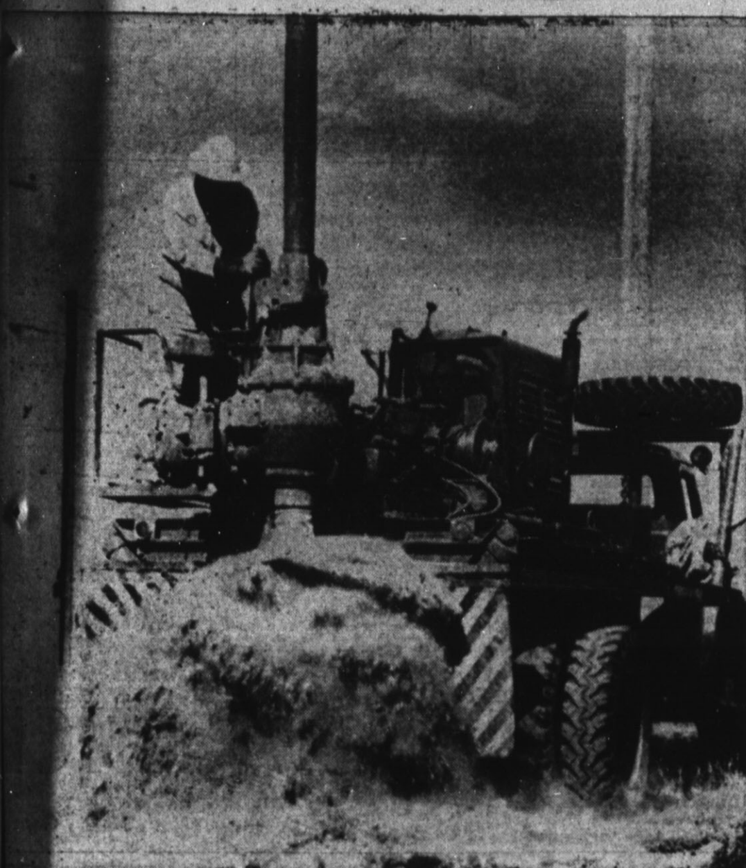
DRILLING FOR POLES —Southwestern Public Service is currently installing new poles along the heavily traveled street. (Staff Photo) needed for changing lighting of Park Ave.
