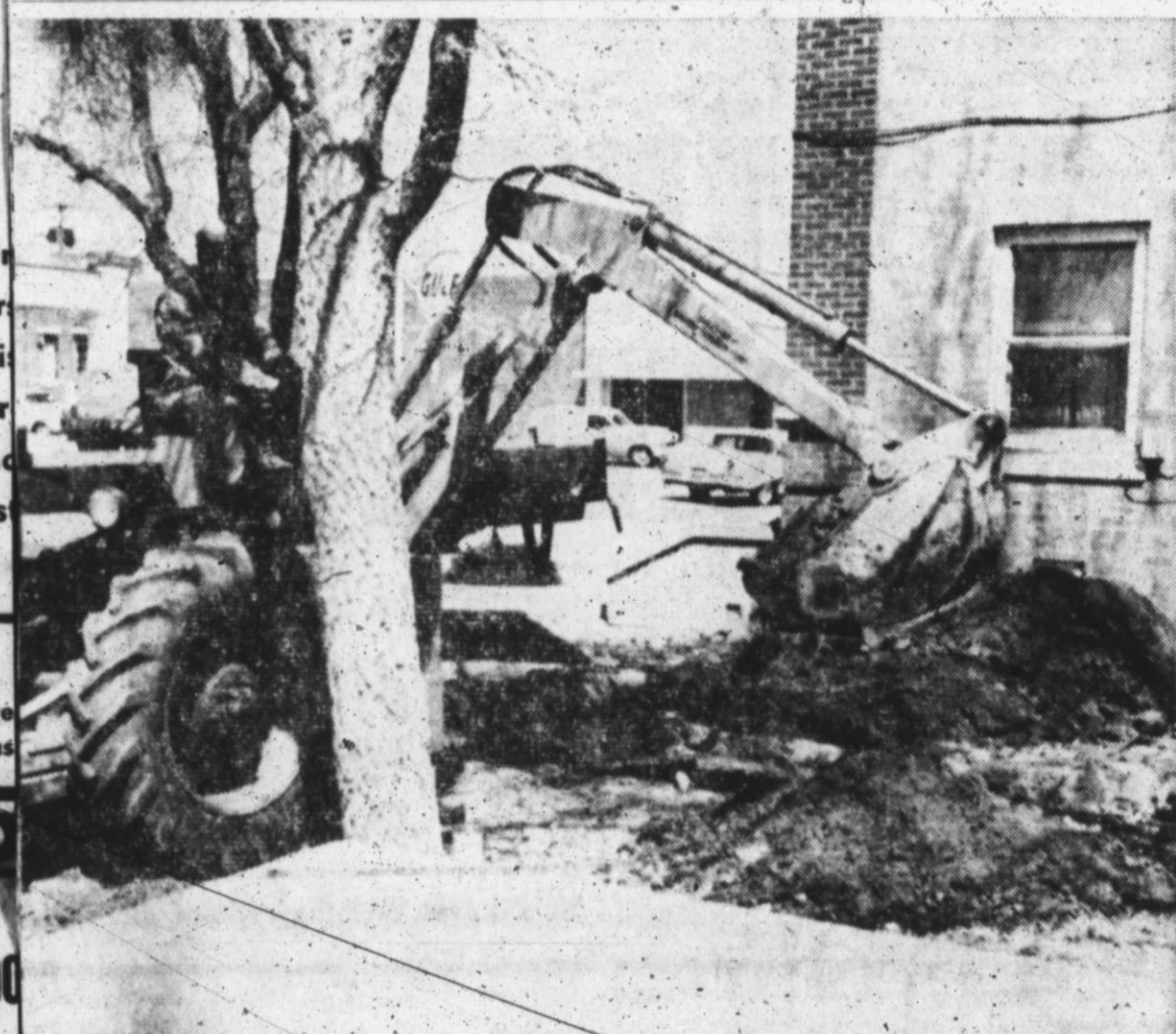
CONSTRUCTION BEGINS — Digging of the foundation to hold two new rooms for the fire marshal's apartment began Monday, the M. B. Allen Construction Co. of Amarillo. Allen won the contract submitting a low bid of $11,459.59. The addition is to be completed within 70 days from the time of beginning. (Staff Photo)
