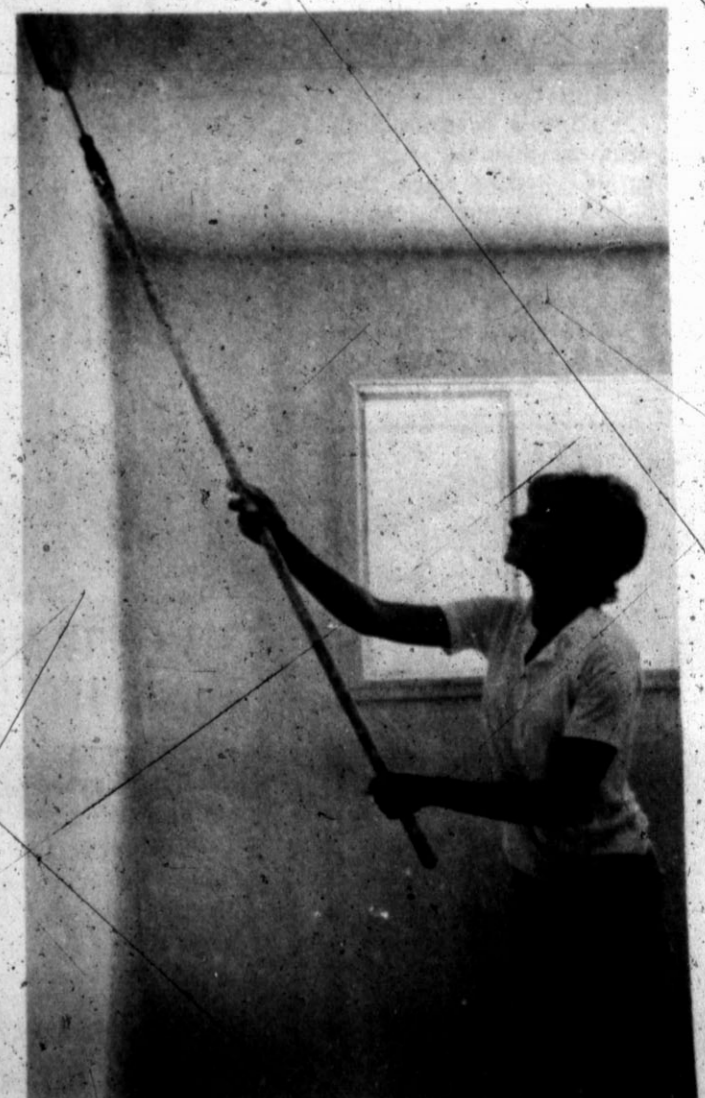
ALL THE WAY TO THE TOP — Mrs. Billy Warrick shortened the stretch involved in painting the high spots in the clinic building.
