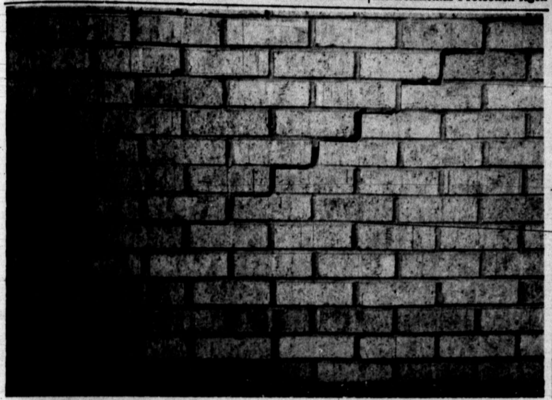
CONSTRUCTION HEADACHE — The crack in this wall resulted in the shrinking and swelling of the soil material of Pullman Clay Loam. This is a problem many builders in Hereford face.
