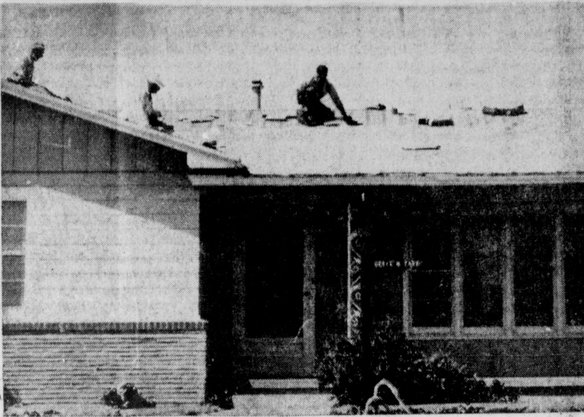
ROOF BUSINESS BRISK — This is a typical scene around Muleshoe these days. Scores of roofs, damaged by spring hails, are being replaced, one insurance man estimating that 20 percent of all roofs were damaged enough to require replac- ing. (Journal Photo & Engraving)
