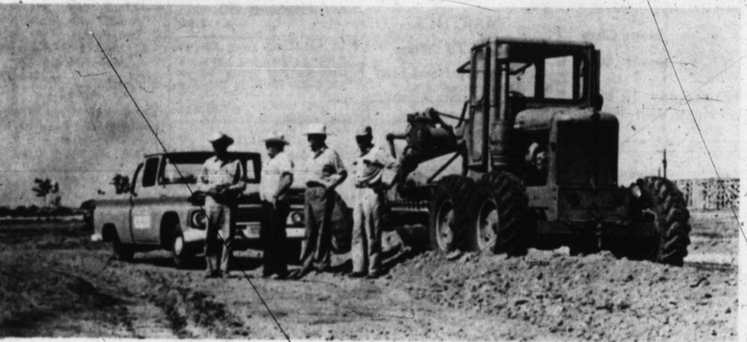
LEVELLING THE LOT that soon will be home of Hereford Masonic Lodge No. 849 was done voluntarily last week by the Tierra Blanca Soil Conservation District. From left are: Ronald Matthews, SCD equipment operator; Blue Turpen, Lodge member; Luther Leslie, SCD board chairman; and Charley Noland, Lodge member. The 160x200 foot
