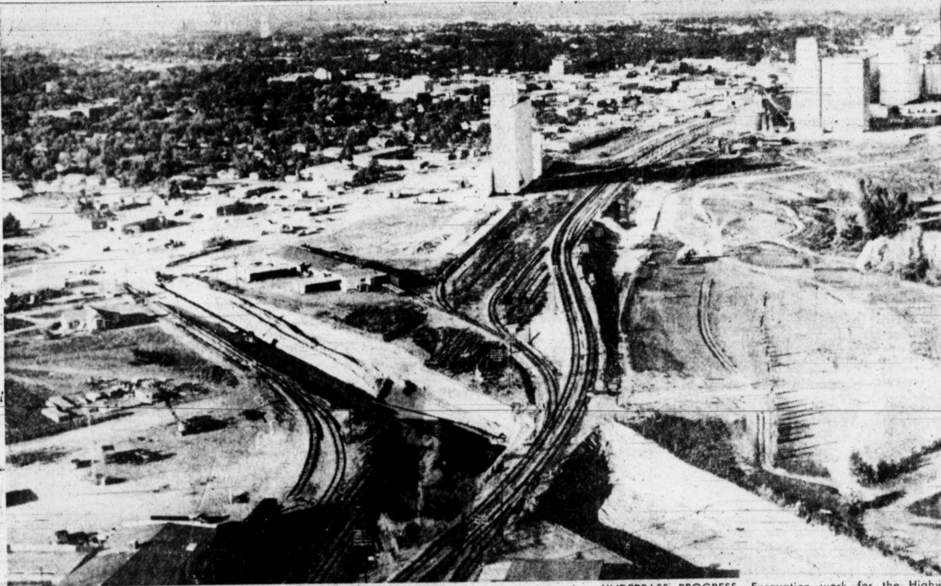
UNDERPASS PROGRESS —Excavation work for the Highway 51 railroad underpass this week made a great slash in the southwest corner of Hereford, above. The main Santa Fe Railway tracks have been cut, with rail traffic continuing temporary on a "shoo-fly" track just south of the area where the underpass will be built. Contractor Ivan Dement is expected to have the work completed "about Christmas" according to a highway department spokesman, with delivery of steel for the job slated for October. (Staff Photo by ROY CLARK)
