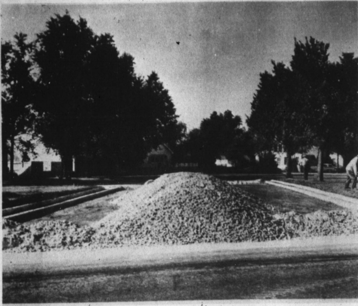
STAR STREET is being extended a short distance south of Park Avenue by street contractors. The tiny street will provide access from Third Street to Star across the tip of the eastern portion of Hospital Park. The street is angled slightly to the south-west from Park Avenue south in order to provide space for several cars waiting to turn. (Staff Photo)
