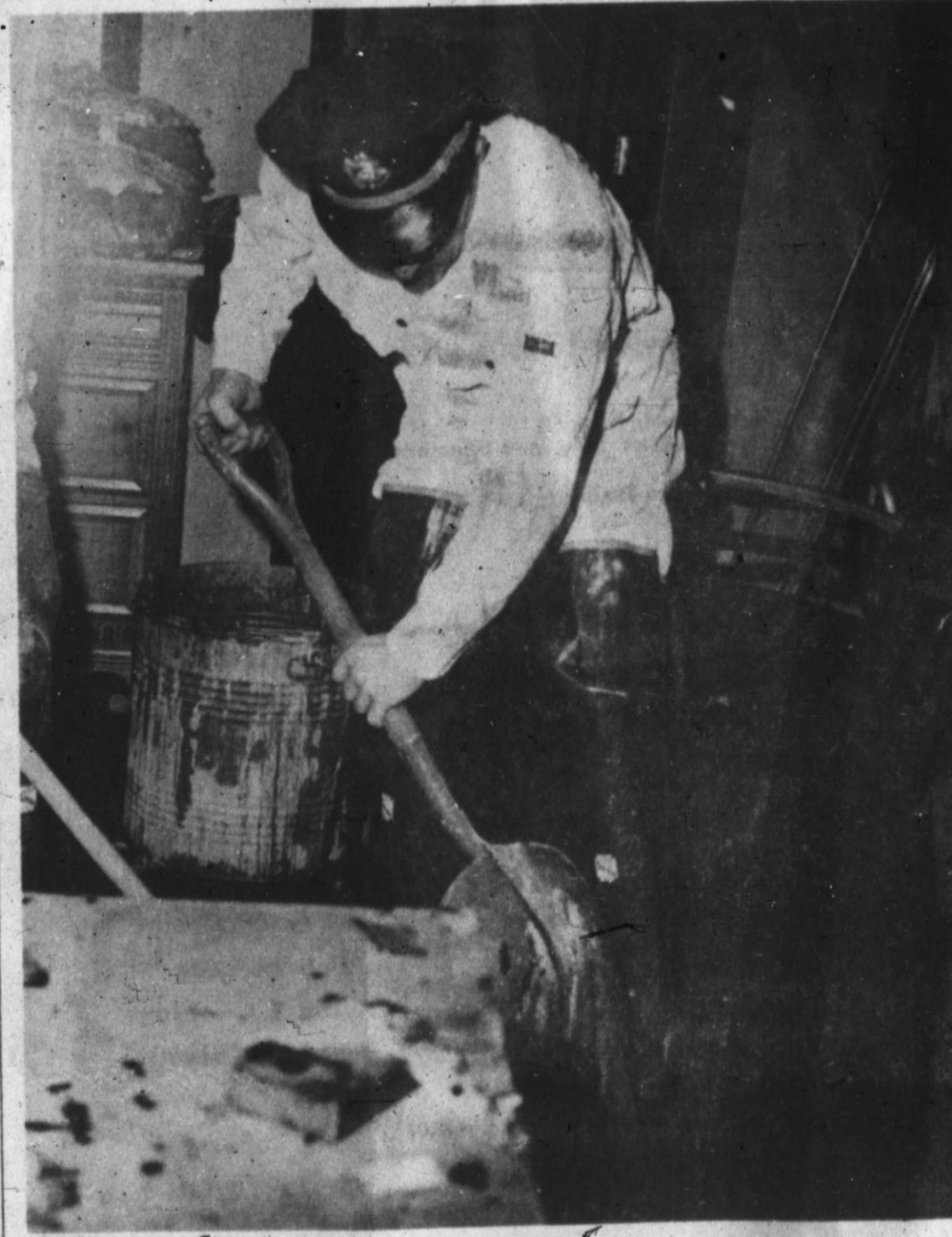
CLEANING UP THE DEBRIS, a Hereford fireman scoops up rubbish after a fire in the Jim Hill Hotel about 9:45 p.m. Friday. Quick work by firemen prevented the fire from spreading to other rooms in the building. The fire was confined to one corner room, with damage estimated less than $1,000. The fire apparently started on a bed in the room but no one was present when fire broke out.
