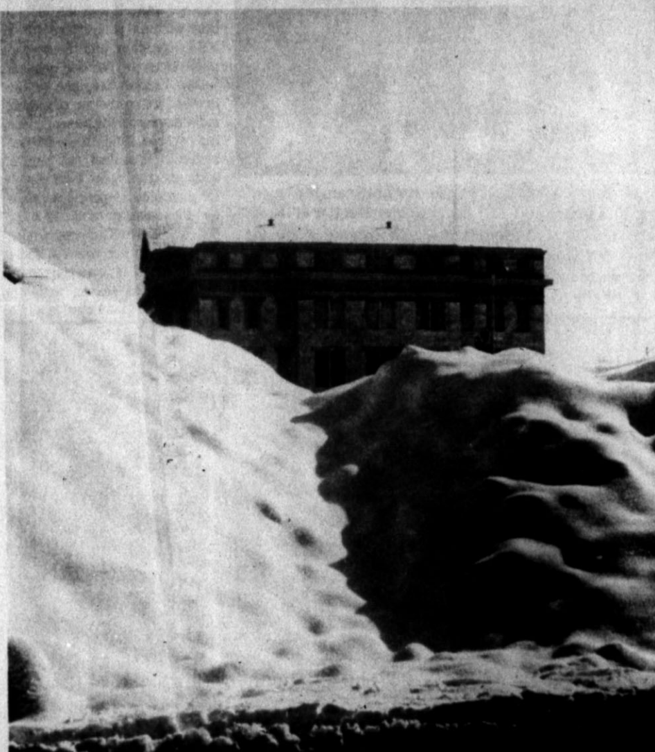
IT PILED HIGH—Though the snow was deep throughout the area late last week, this picture tends to exaggerate the depth. Actually, snow covered the mounds of dirt piled high near the construction site of the First National Bank, seeming to "bury" the courthouse in the background.
